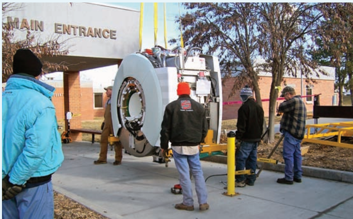
A crane was used to hoist Clay County Medical Center's new MRI unit through the main entry of the hospital in January.
